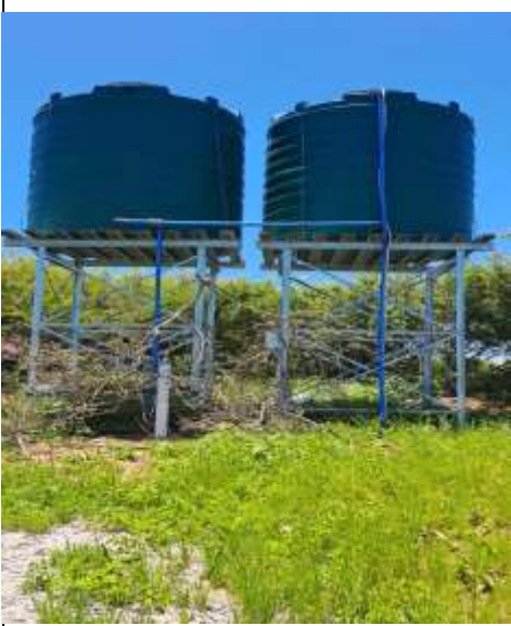
▪ Water reservoirs linked to a borehole
